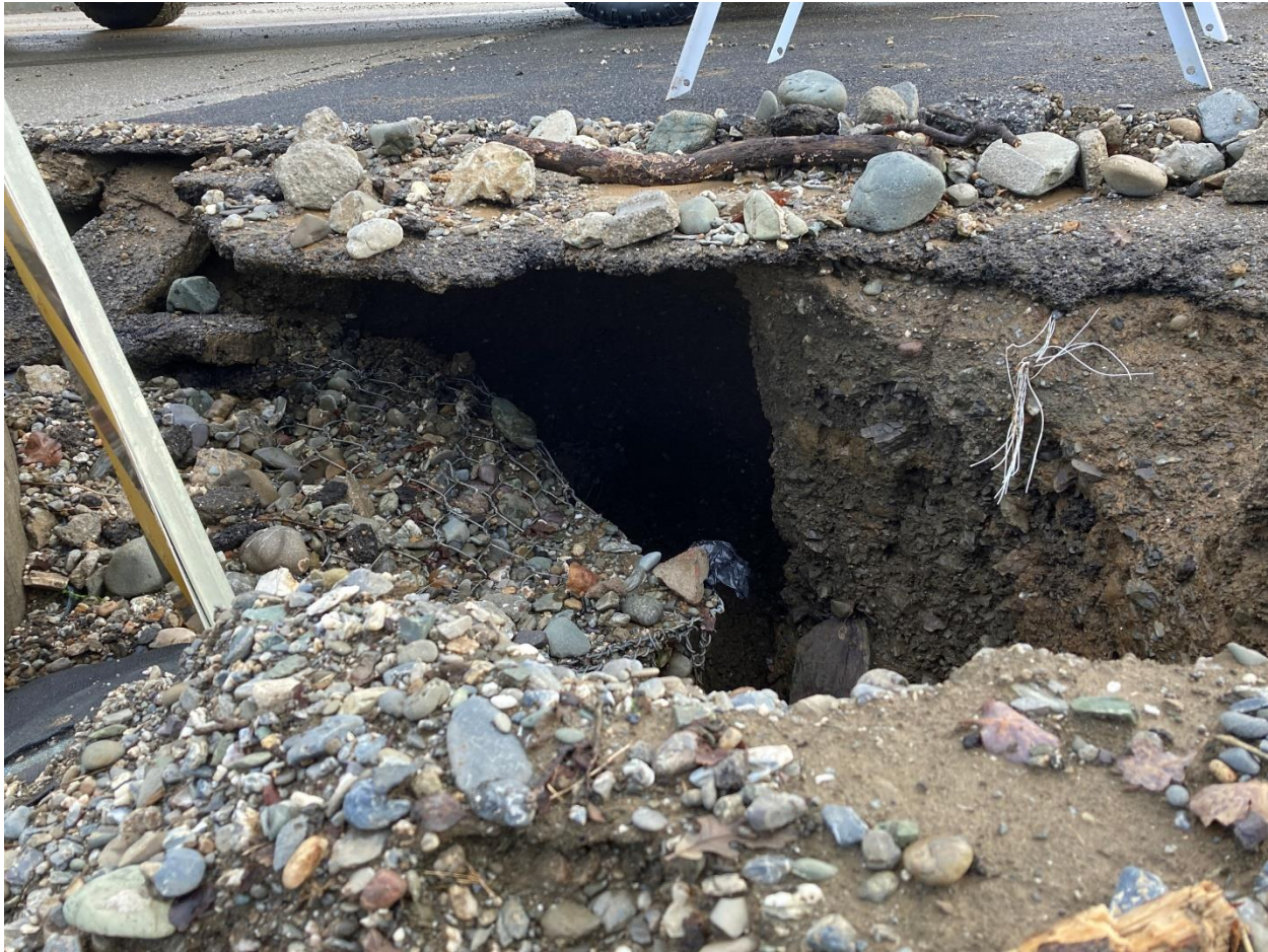
Figure 5 - UNDERMINING OF BRIDGE APPROACH
